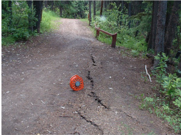
Figure 13 Tension cracks in the lower trail
